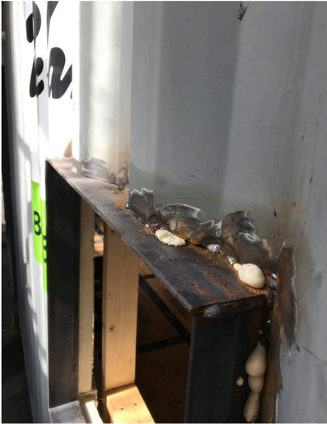
Figure 3. Challenging window openings. Photo by author.
